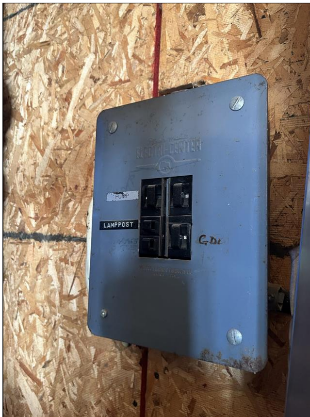
7.3 Item 1(Picture) panel conditions
