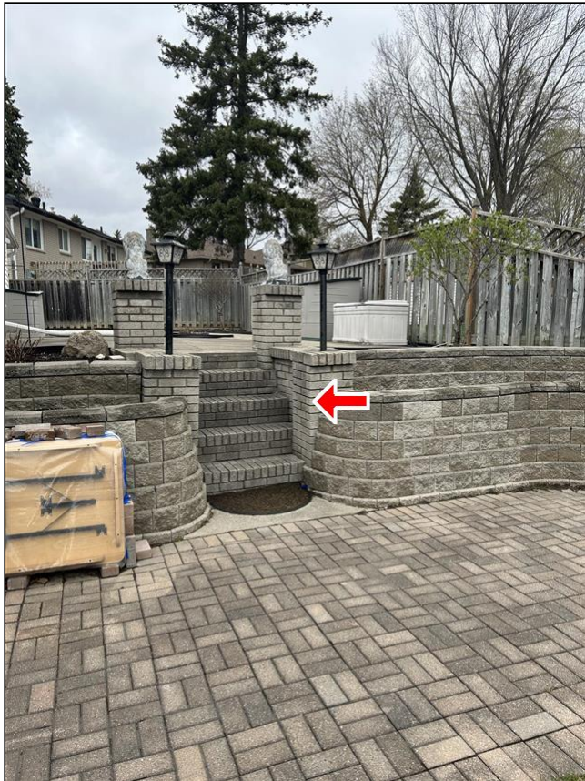
1.11 Item 1(Picture) missing railing
