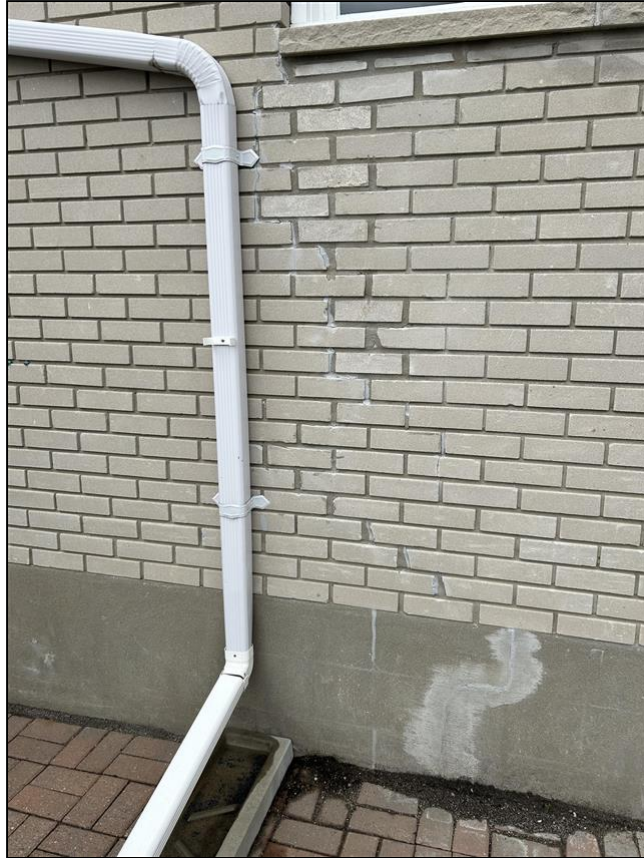
3.0 Item 1(Picture) step cracking
