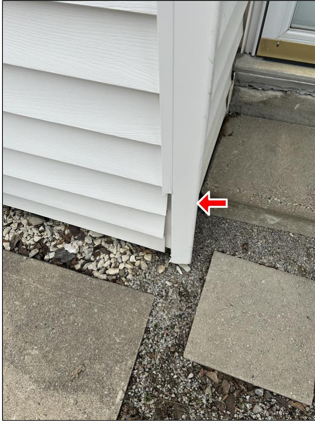
1.2 Item 1(Picture) damaged siding
