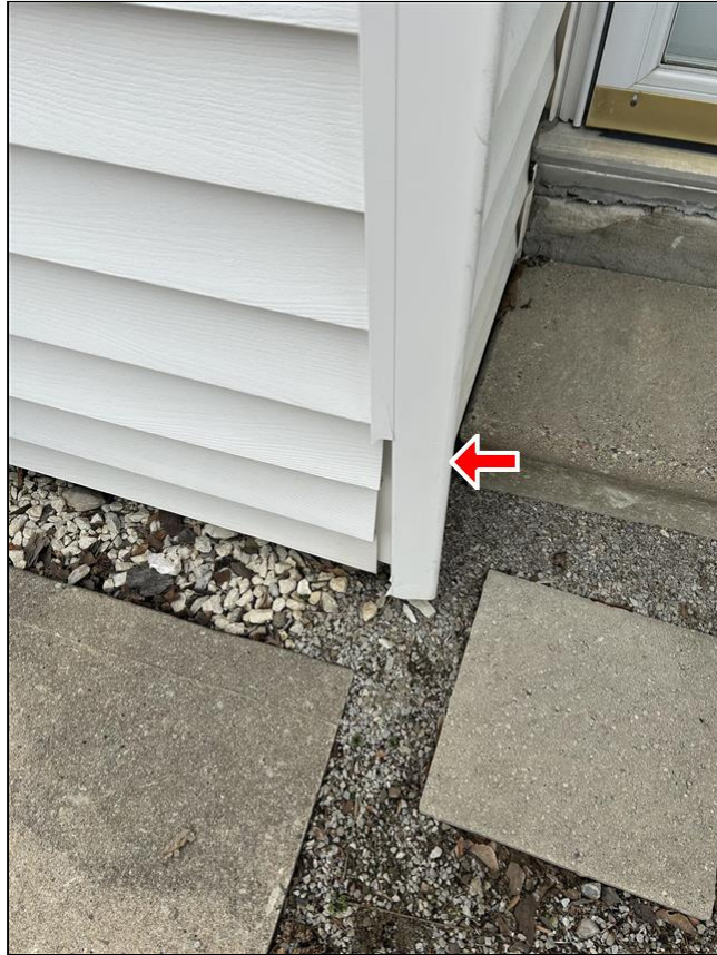
1.2 Item 1(Picture) damaged siding
