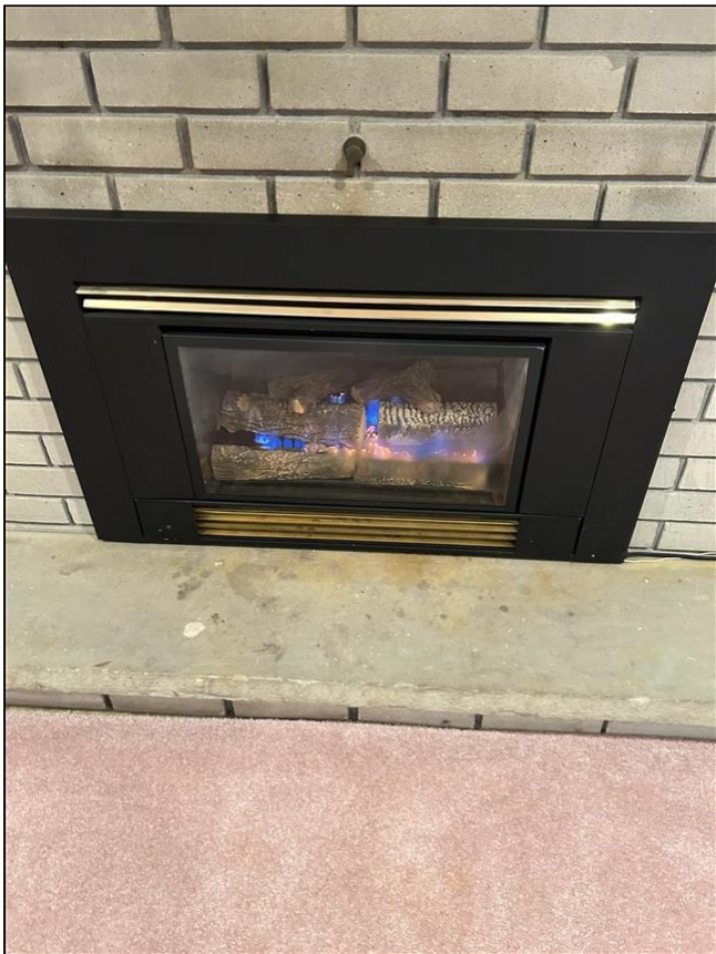
14.8 Item 1(Picture) gas fireplace condition
