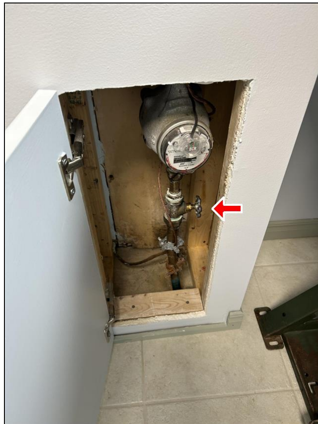
6.0 Item 1(Picture) main shut off
