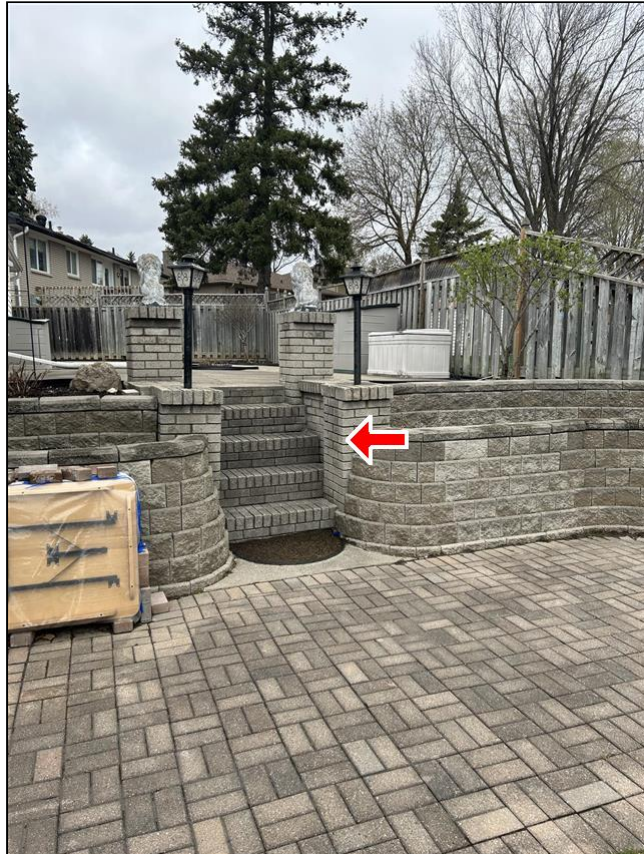
1.11 Item 1(Picture) missing railing
