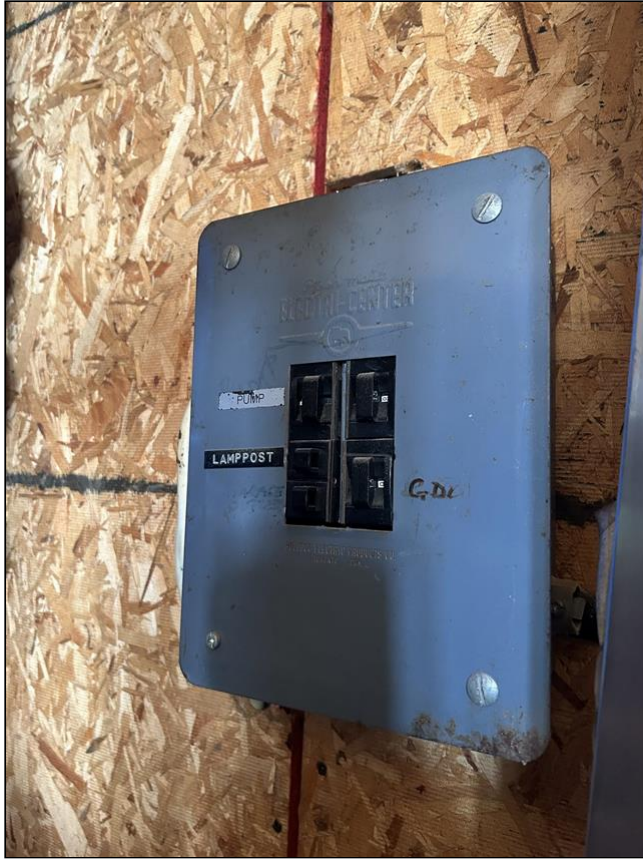
7.3 Item 1(Picture) panel conditions
