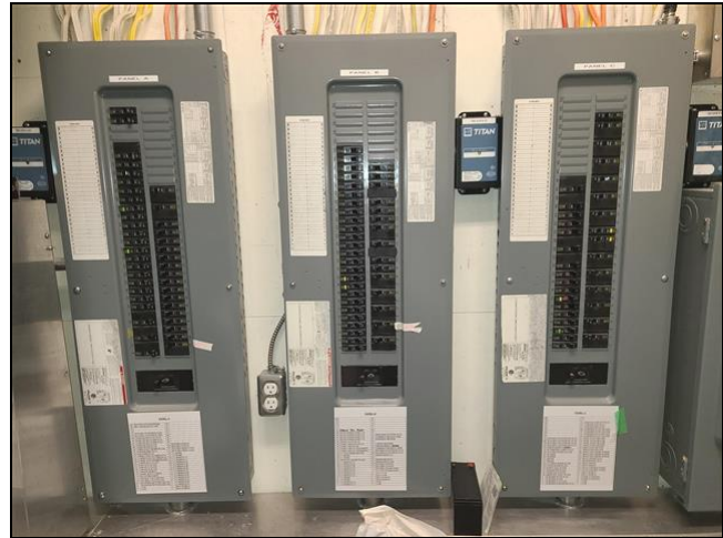
Main House Panels
