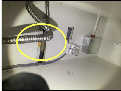
12.14 Item 2(Picture) Gas Stove Shutoff Valve
